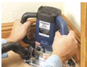
Undercuts Inside Corners
